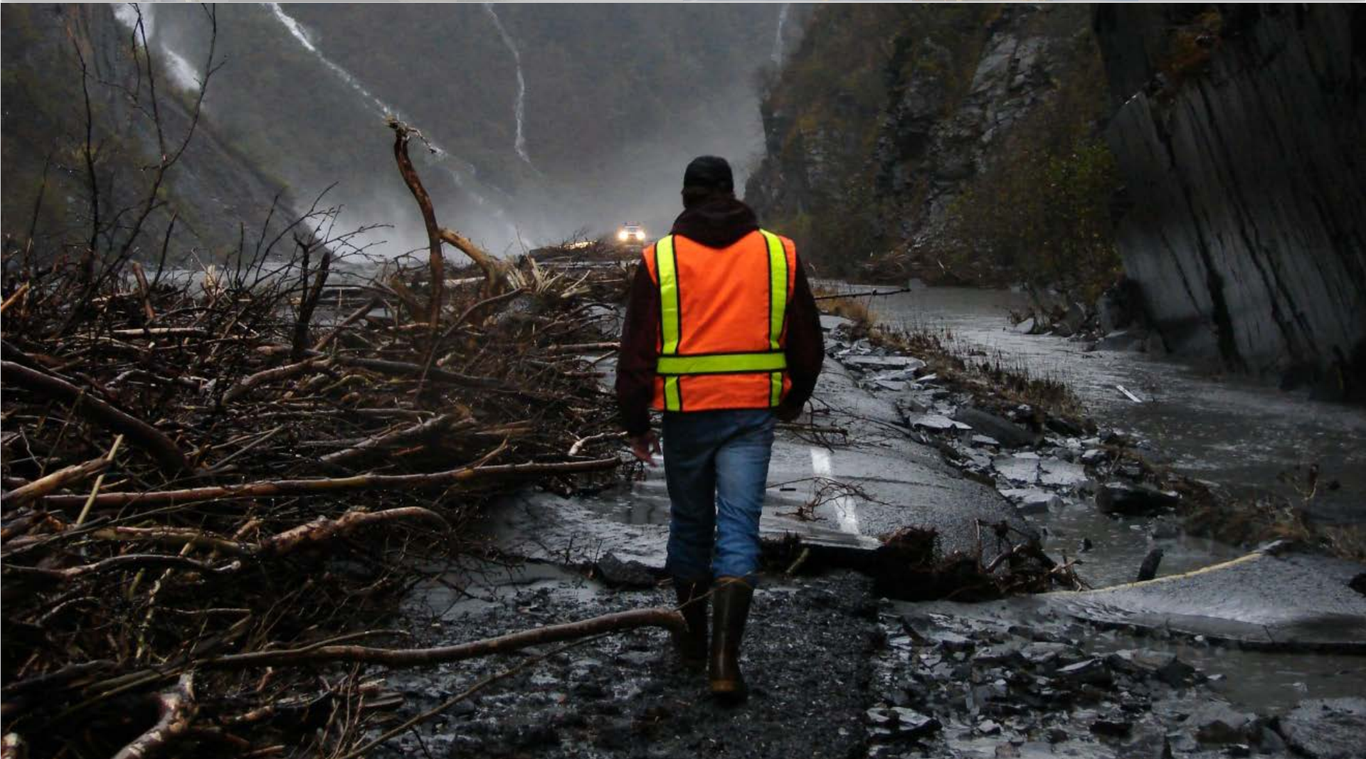
Assessing flood damage on Richardson Highway in Keystone Canyon. Photo by Mike Isaacs, Alaska DOT&PF
