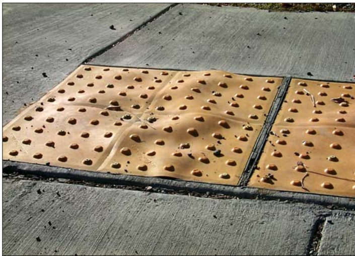
Installation 2: Close-ups of lost adhesion under mat at and edges.
