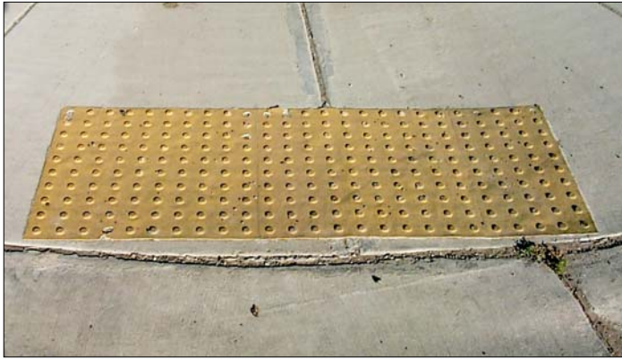
Installation 7: Located on the northwest corner of the intersection of 3 rd Ave. N. W. and 6 th St. N. W.
