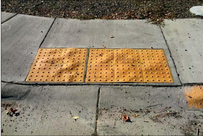
Installation 2: Located on the southwest corner at the intersection of 6 th Ave. N. W. and 6 th St. N. W.
