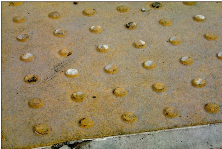
Installation 7: Close-up of damaged mat. Loss of domes and torn surface.
