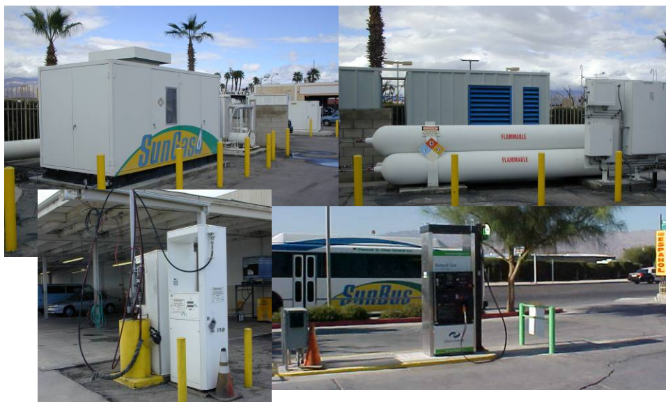
Figure C-4. CNG fueling equipment (Indio)
