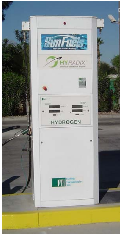
Figure C-8. Hydrogen dispenser at SunLine
